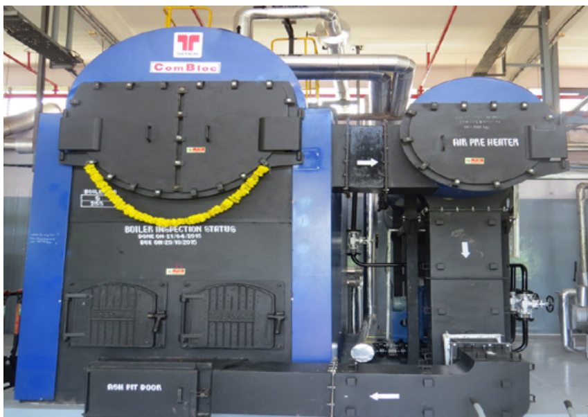
Photo: Solid fuel (Biomass) Boiler, Teva, Goa.
